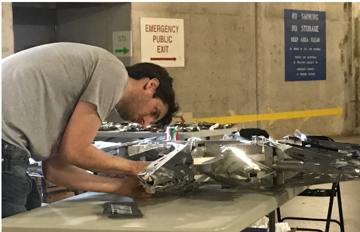
Technical Director Jeff Collier preps the internal wiring harnesses prior to installation.
