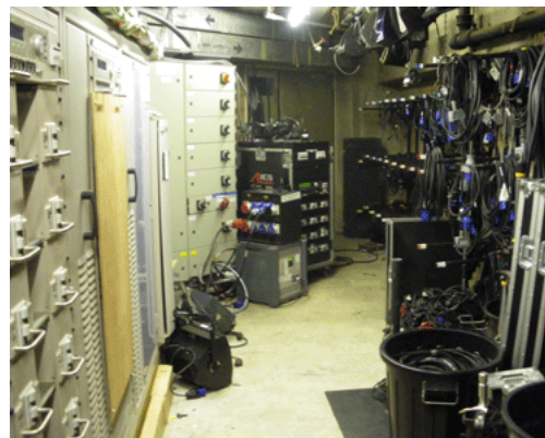
New IES dimmers being installed
