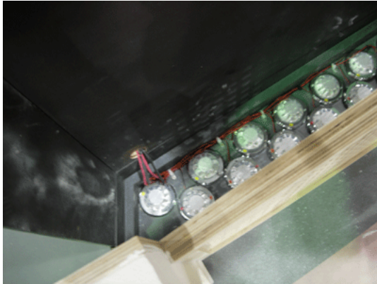
A detail here of the Fireplace LEDs from the Nursery Set. These are Jumbo LEDs from http://autolumination.com - they're used as truck back-up and dome lights and come in orange and red. They're powered by batteries built into the set piece along with a SHoW DMX Receiver and SHoW DMX Dimmers.
