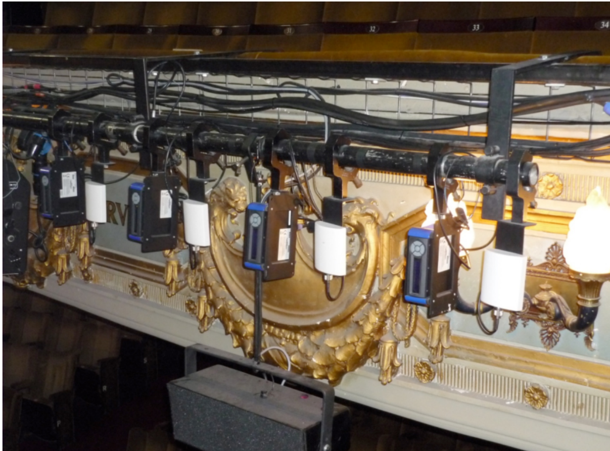
Transmitters and Panel Antennas on Circle Front
