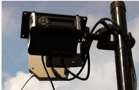
Close up of a SHoW DMX Receiver with a panel antenna.
