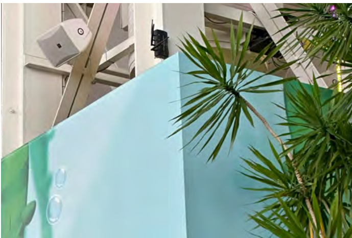
American Dream's Nickelodeon Theme Park includes Multiverse Transmitters to transmit wireless DMX to the QolorPIX Tape Controllers controlling the QolorPIX Pixel Tape vertically applied to the main beams
